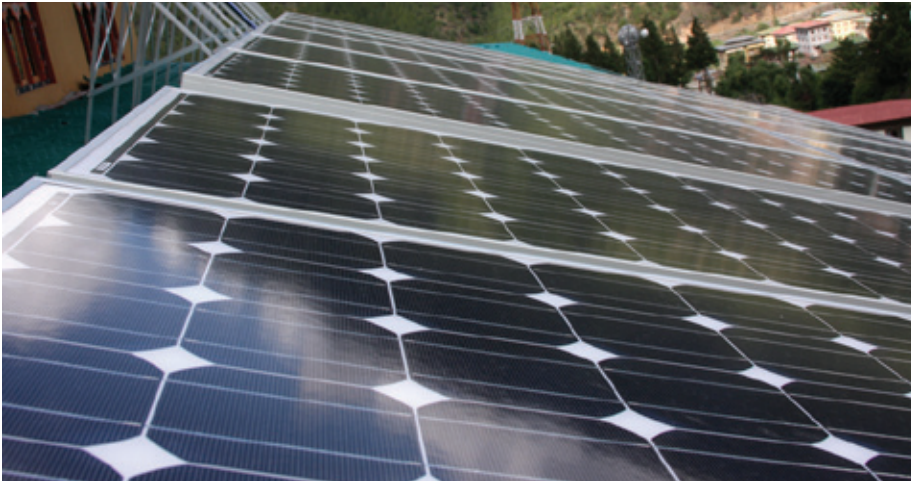
Solar panels installed on RSPN headquarter's rooftop
