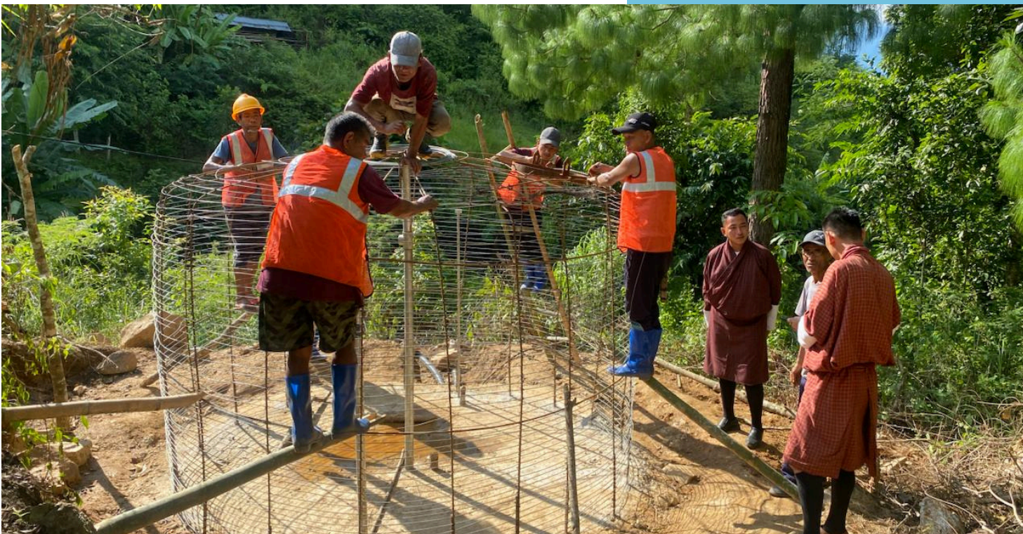
Construction of water reservoir tank as part of RWSS at Tsholingkhar Gewog, Tsirang.
