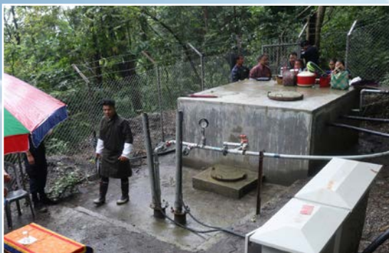
50,000 liter capacity submersible pumping system station and collection tank at Dumsidara
