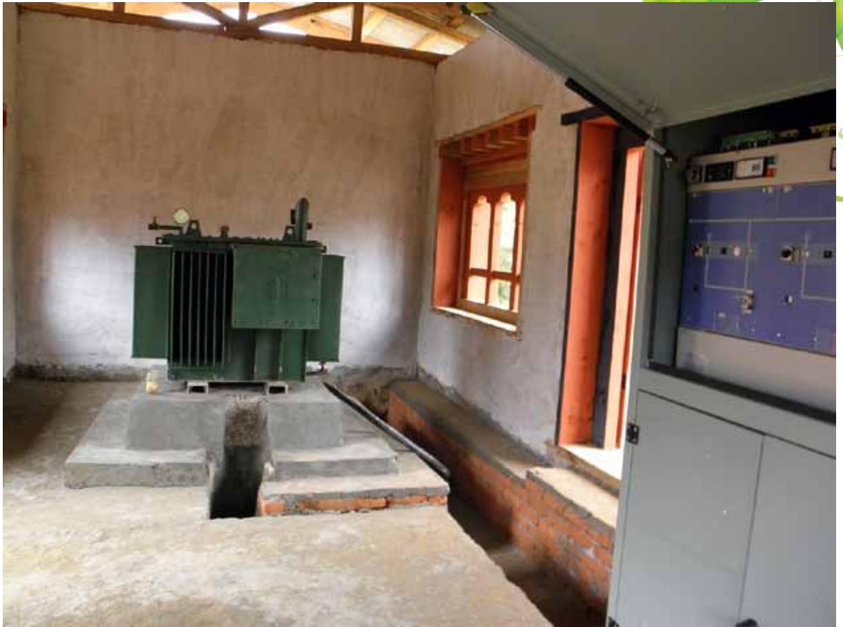
Transformer installed inhouse to prevent any casualties for cranes
